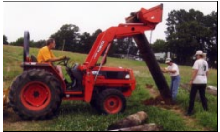
Rick Richardson, Brynda Read, and Peggy Hart working on the large drop at the Cross Country Course. Due to equipment malfunction, this project will have to be completed this fall.
